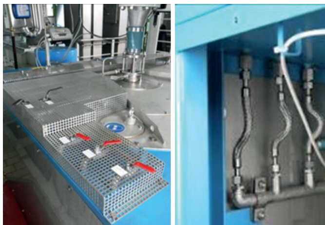
Figure 13: (left) central water and steam supply, (right) stainless steel piping
